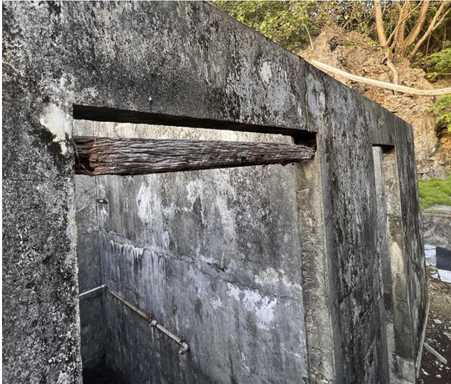
Figure 6: Close-up of dropped lintel to R3 doorway.
