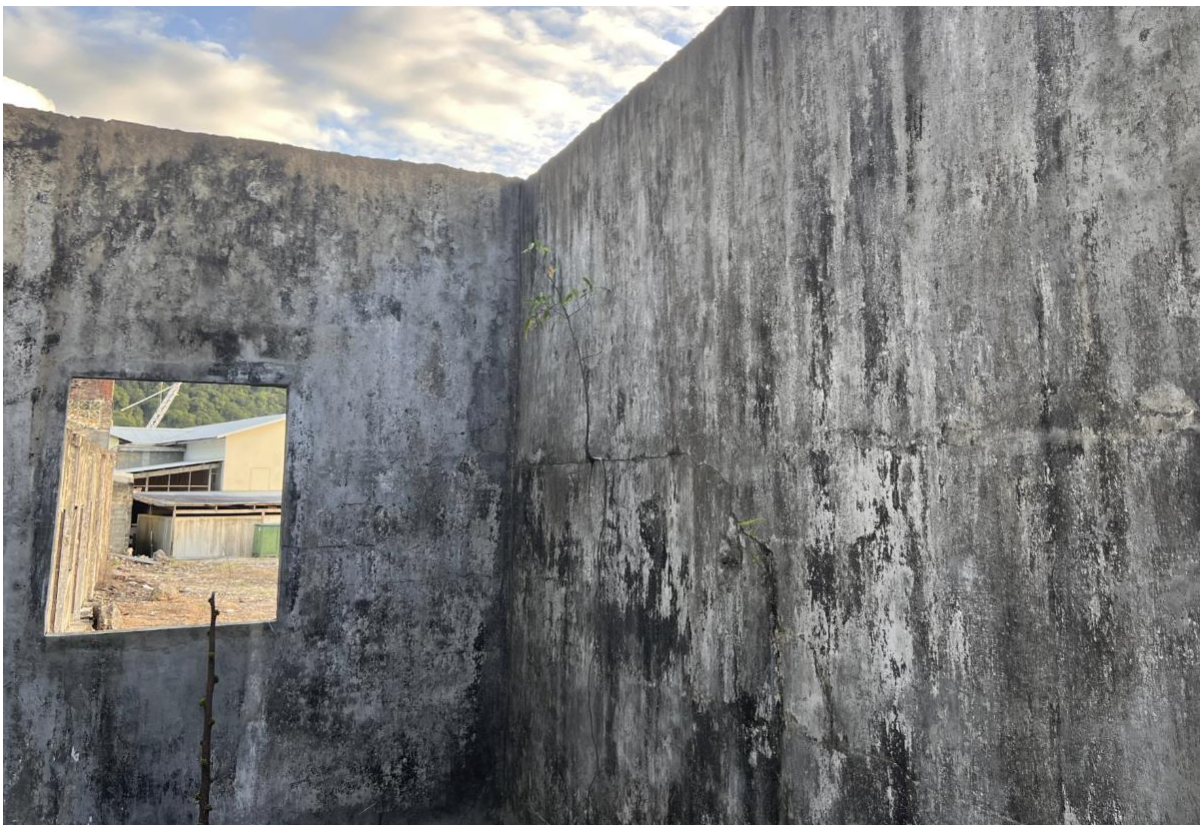
Figure 3: Plant growth occurring at cracks to internal wall. Separation cracking at the return external wall is also visible.
