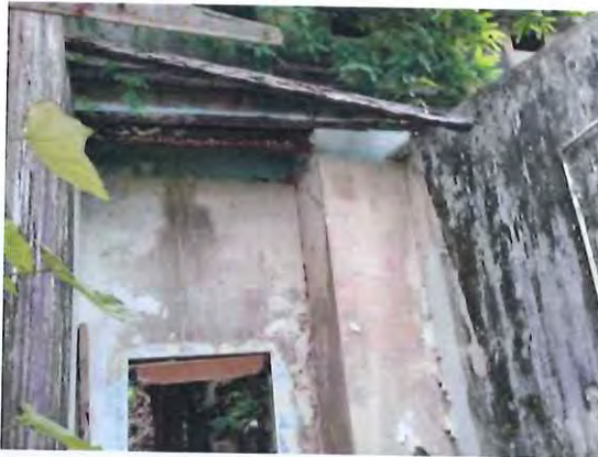
Figure 2.6 Missing roof to the first floor. (Source: Inter Engineering, 2018)
