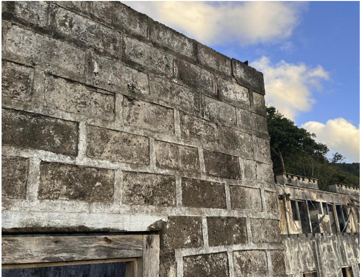
Figure 2: Loose brick at upper corner of front elevation.
