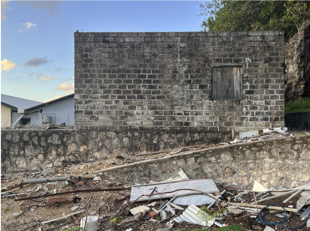
Figure 4: External elevation, showing missing window frame, and also vertical cracking coinciding with return wall.
