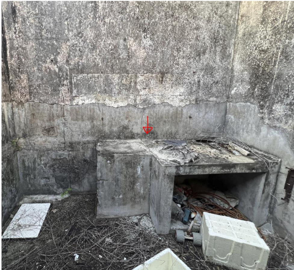
Figure 8: View showing lower return nib wall coinciding with crack visible in Figure 7.
