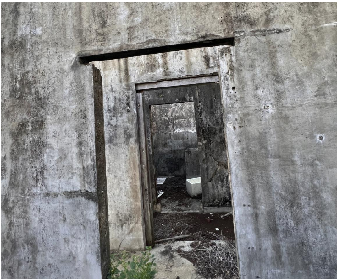
Figure 5: View showing two missing door frames (fore ground and back ground). Note the horizontal crack extending from lintel level to the door frame in the fore ground.
