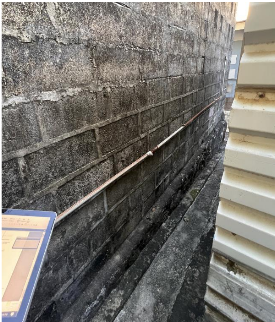
Figure 7: Vertical crack visible on external wall of Elevation 4.
