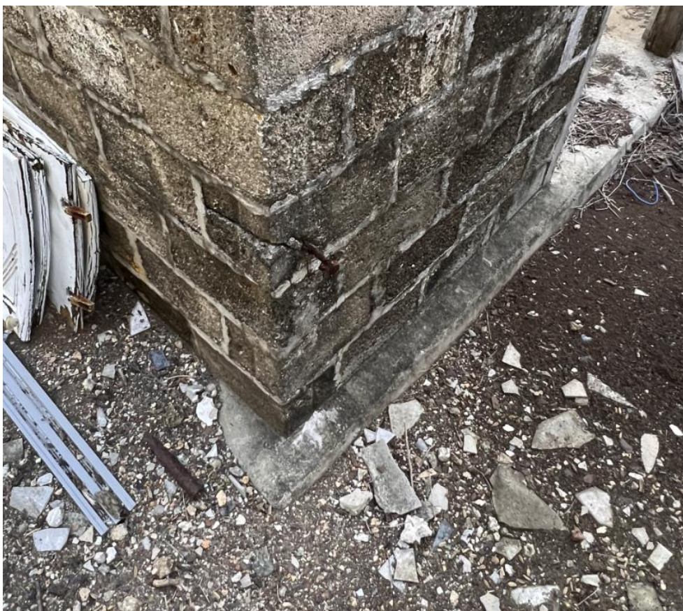
Figure 9: Cracked brick to corner wall, caused by corroding embedded anchor.
