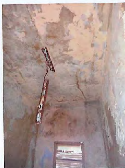
Figure 2.11 Detail of room interior showing substantial deterioration. (Source: Acker Pty Ltd, 2017)
