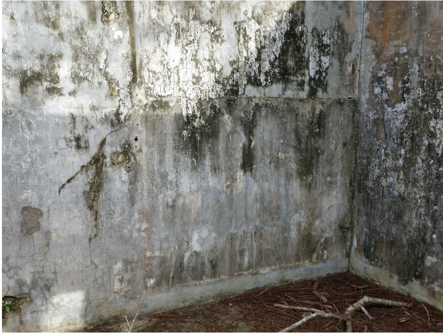
8. Internal walls - cracking
